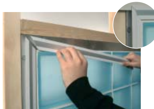
Step 5 : If using plasterboard coverstrip carefully measure, mitre corners and slot into position.
